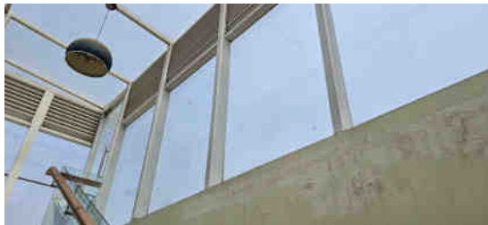
Figure 22. Louvres windows used as outlet openings Source: author, 2025
