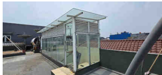
Figure 20. Solar-induced glass room chimney Source: Author, 2025
